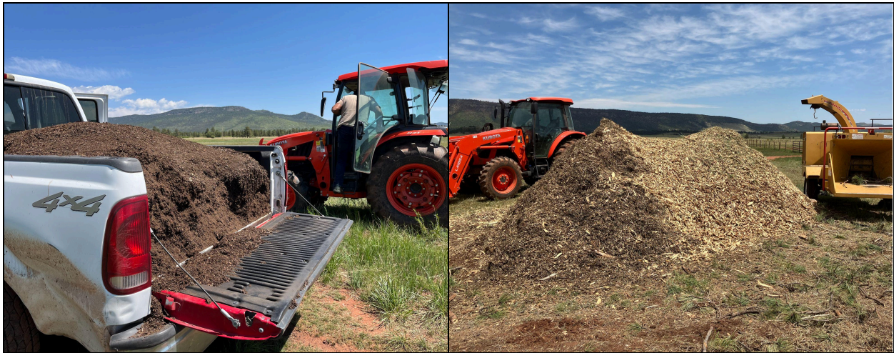
Figure 3: Left: Truck loaded with approximately 1-1.5 cubic yards of compost. Right: Mulch pile ready to be applied to site
