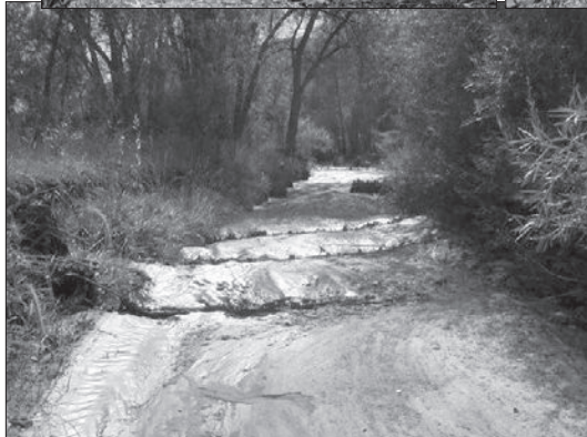
Working in the Galisteo. [Top] Galisteo Creek before. [Middle left] Wicker weirs installed. [Middle right] Weir close-up. [Bottom] After the first flood event.
