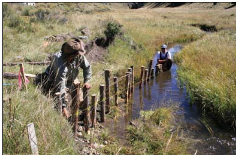
Volunteers construct bank stabilization structures called post vanes to help restore resilience to Comanche Creek, Valle Vidal unit of the Carson National Forest, NM, September 2007. (photo by T. Gadzia)
