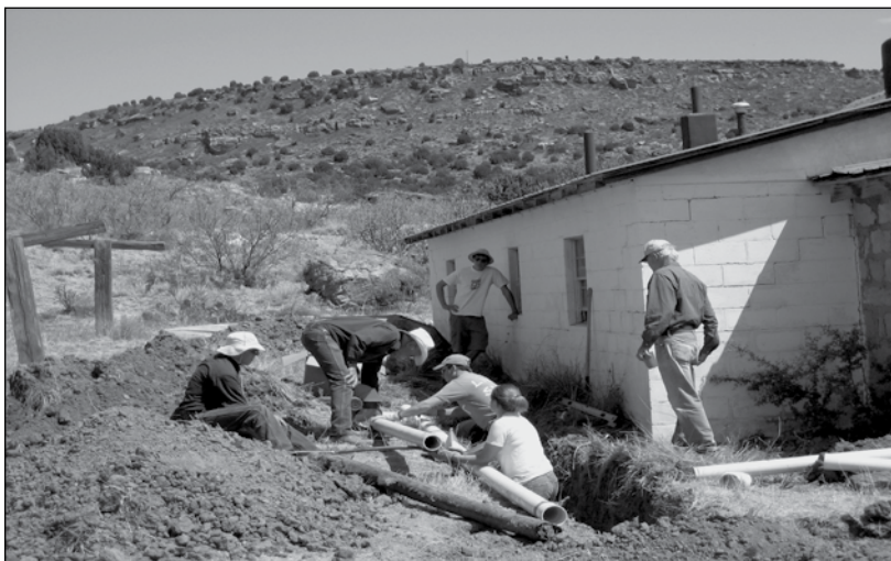
Family members installing a new septic system for the bunkhouse during the 2006 work week.
